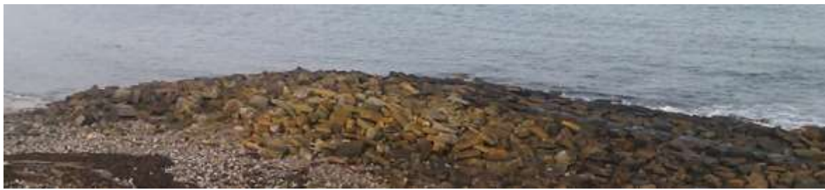
Figure 2.30 Collapsed breakwater at Skateraw (2014)
