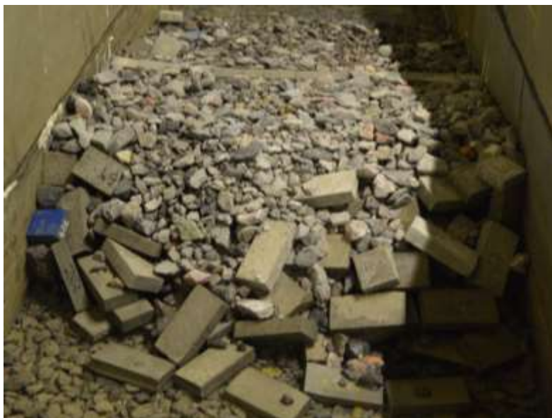
Figure 7.14 Series 2, post collapse, view from leeward
