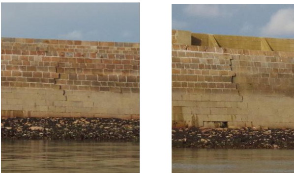
Figure 14 Cracks are beginning to appear in the south face of the wall
