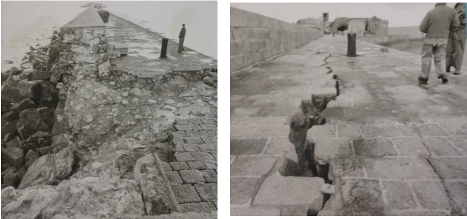
Figure 12 Breach in the parapet and longitudinal fissure, 1978
