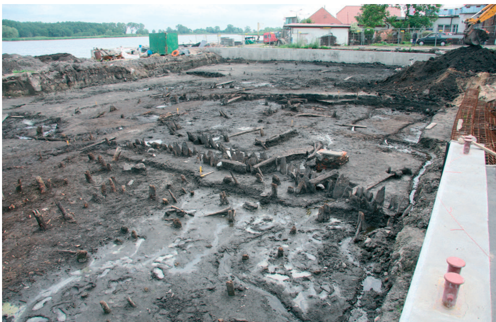
Fig. 11. Wolin, site 3. Central quay in palisade construction – view from the northwest. Photo A. Janowski
