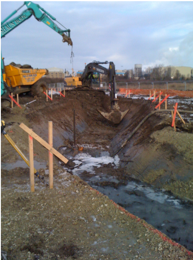
Fig 1.3 Photograph showing the challenging site conditions of the watching brief on the new compensatory watercourses in Kemsley Marsh
