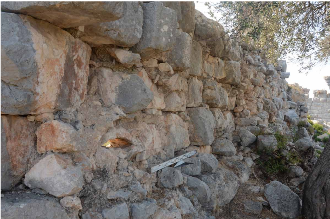
Figure 23. A part of the Late Antique City Wall. The ashlar blocks of the outer shell are not truly connected to the filling (@ Patara Excavation Archive).
