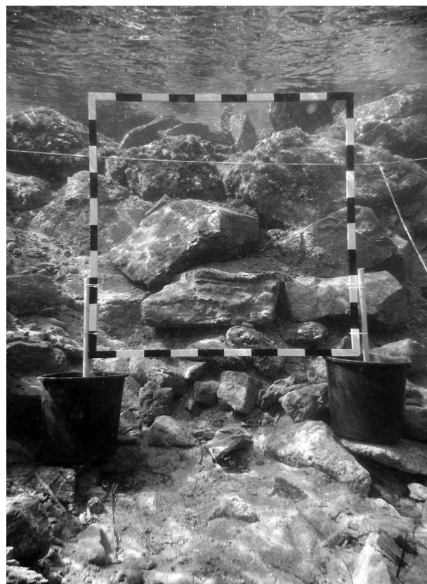
Figure 16. View of the lower courses and foundation level for the western mole in L2 during excavation of Trench 4 (T. Nowak).
