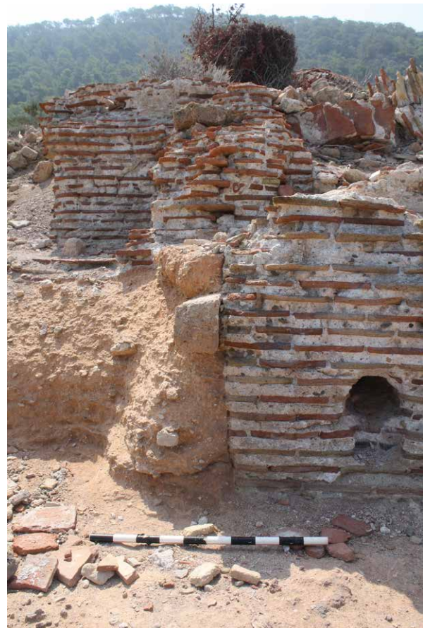
Figure 9. The surviving brick structures, which were not robbed for building material, provide a clear illustration of how many of the rock cuttings along Dana's shore were used as building foundations. The foundation here is cut into the more friable stratum below the quarried layer (Photo M. Jones).
