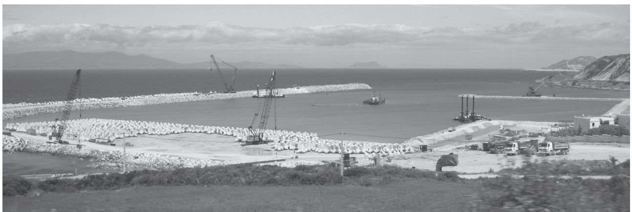
FIG. 47. (BELOW) “BASE NAVALE DE KSAR-ES-SEGHIR” DURING ITS CONSTRUCTION, 2009. THE REMAINS OF WHAT WAS THE SITE OF ZAHARA ARE JUST AT THE RIGHT EDGE OF THE PHOTO (PHOTO: AT).
