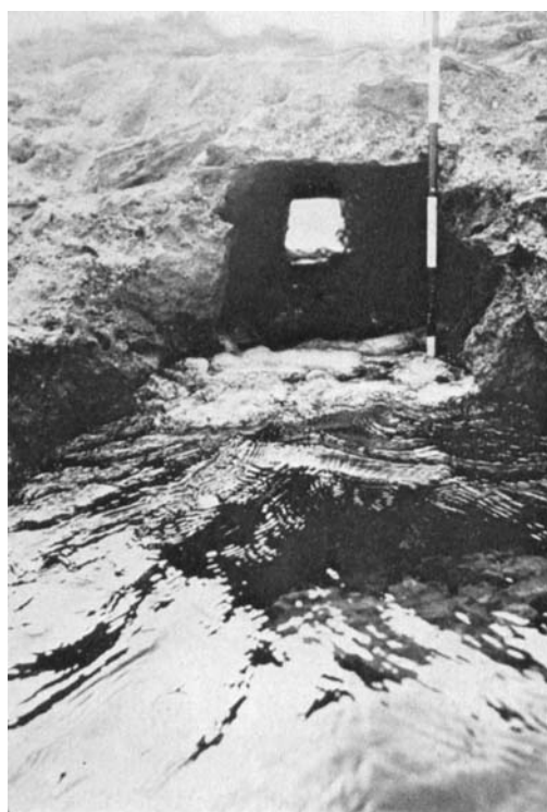
Figure 7. The original location of a wooden former in the concrete platform in front of the Neptune restaurant.
