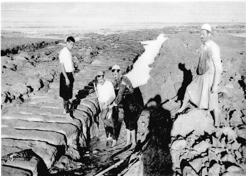
1. Attempt to find the depth of the foundation of the land leg of the breakwater.
