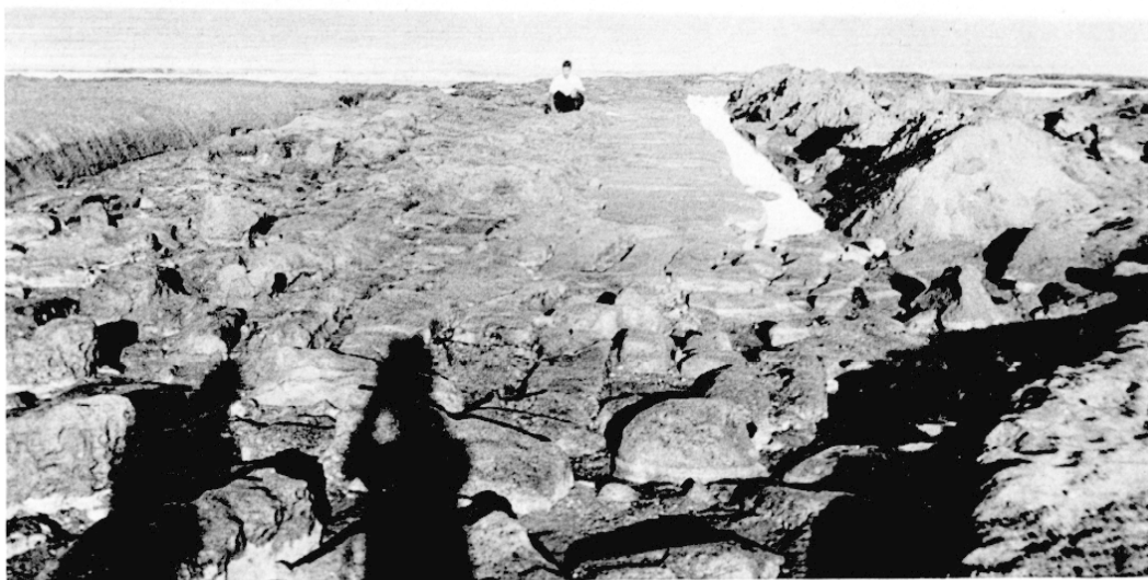
2. The land leg of the breakwater, with the smoothed tumbled stones in the foreground.
