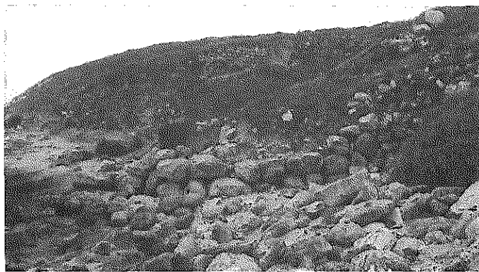
Photo 9.43. The retaining wall at the southern side of Tel Dor, looking northwest.
