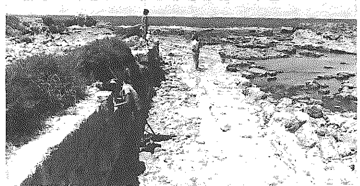
Photo 9.16. Flushing channel 2, looking west. The surveyor on the right stands on the pre-existing quay, facing another who stands on top of the southern side wall.
