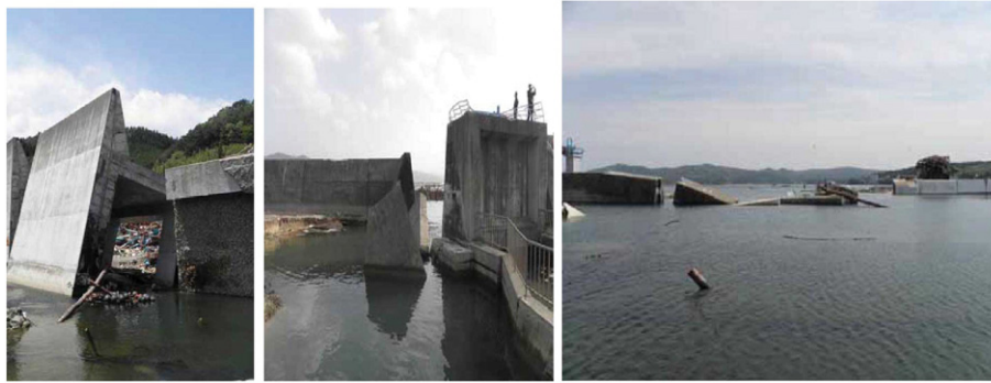
Fig. 7. Photos of damaged cement harbor foundations at Kojirahama (Top left), Utuchi (middle), and Tanesashi (right), Japan following the March 11, 2010 Tohoku-Oki great earthquake (from Ewing, L.: from Lesley Ewing, Sr. Coastal Engineer California Coastal Commission, "Port & Harbor Damage from the March 11, 2011 Tohoku Oki Tsunami", www.coastal.ca.gov/nps/Tsunami_Lessons.pdf ).
