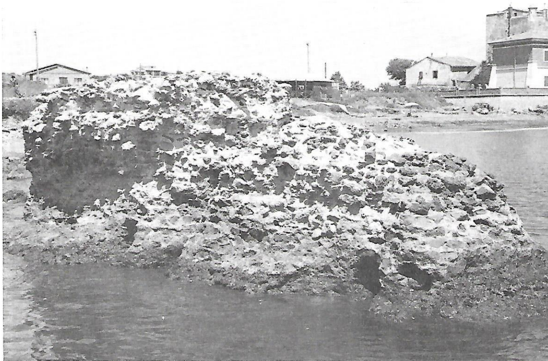
30. Concrete Pier 2, harbour of Cosa, showing holes left from strengthening crossbeams in concrete.
