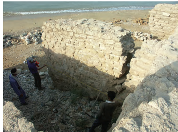
Figure 5. A seaward-facing buttness (marked with an 'X' in Fig. 4) on the southern side of the Congregational Mosque (Site B) clearly showing the impact of erosion. (Photo: A. Trakadas)
