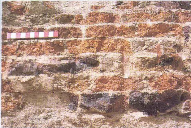
B. Kamrej: Burnt brick structures set in coarse lime mortar. 1st-2nd century A.D.
