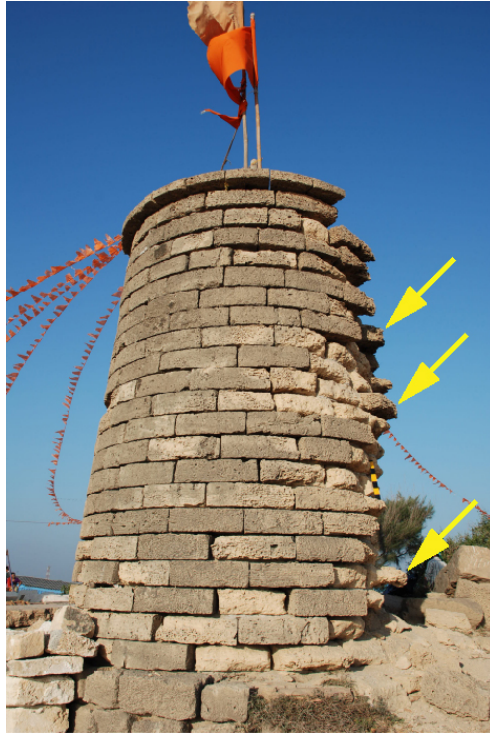
Figure 3. Arrow marks indicating the damaged projecting steps to climb on the top of structure (Photo: Sundaresh).
