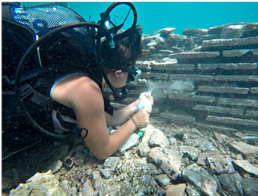
Fig. 16. The filling on the upper masonry surfaces carried out using the supply pockets made of a waterproof fabric (photo ©ISCR).
