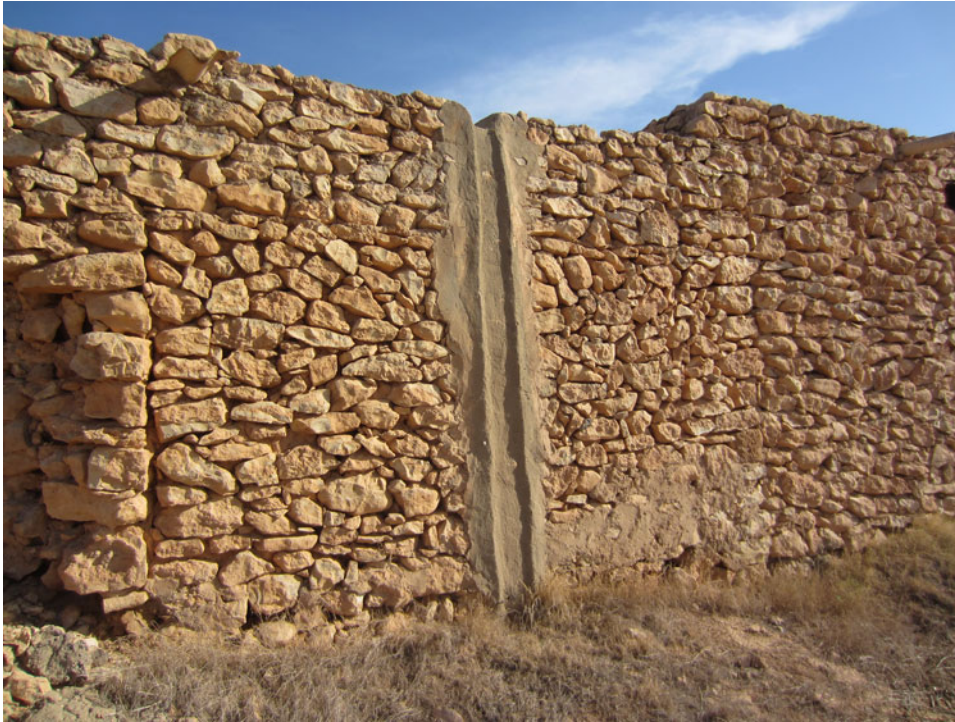
Figure 42. Plaster vertical strip used as a downpipe (KHM 161). Photo: Archaeological Mission Roma Tre University. (Colour online.)
