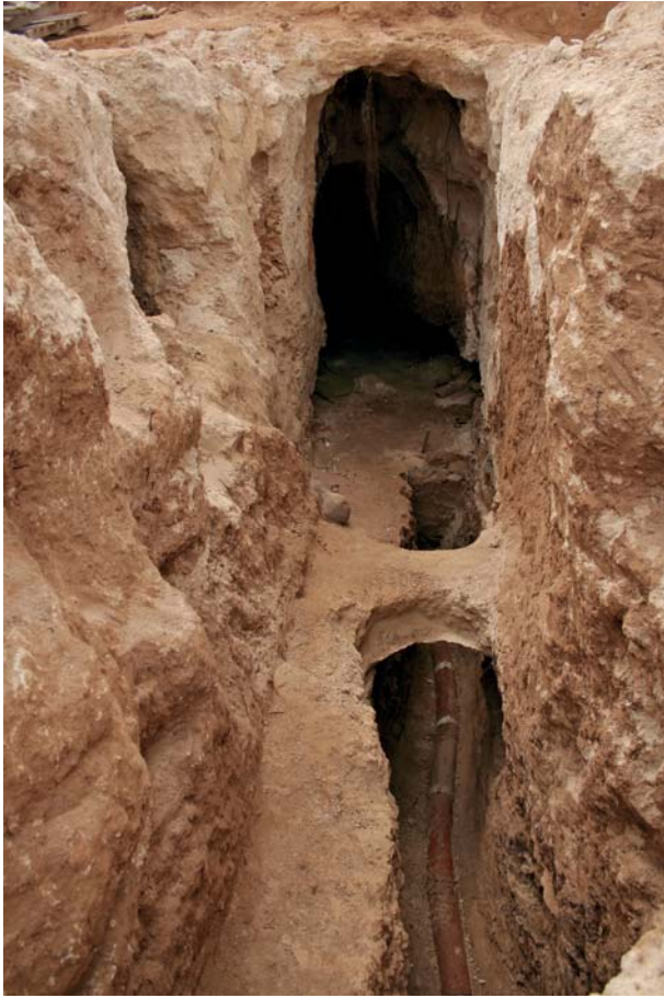
Fig. 24. Tunnel dug into the limestone for laying the pipes of a water main.
