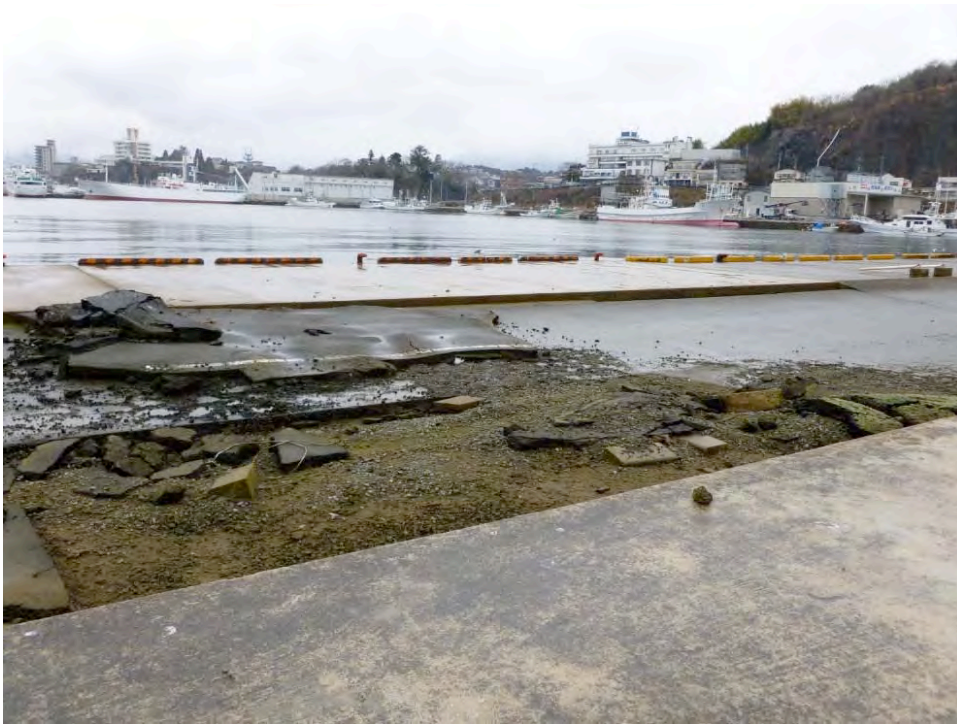
Figure 2 – Pile-supported dock with local subsidence failure of dockside infill: Kesenuma Port, Japan, March 10, 2012, one year after tsunami.
