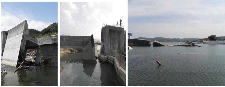
Fig. 7. Photos of damaged cement harbor foundations at Kojirahama (Top left), Utuchi (middle), and Tanesashi (right), Japan following the March 11, 2010 Tohoku-Oki great earthquake (from Ewing, L.: from Lesley Ewing, Sr. Coastal Engineer California Coastal Commission, "Port & Harbor Damage from the March 11, 2011 Tohoku Oki Tsunami", www.coastal.ca.gov/nps/Tsunami_Lessons.pdf ).
