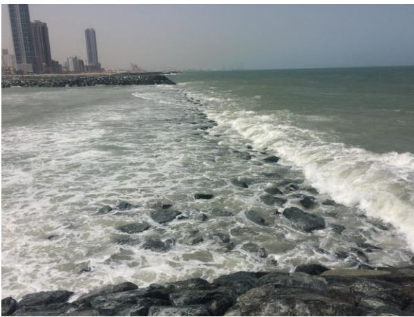
Figure 10 Photo of performance of submerged breakwater during low tide (0.1m LAT) with wave breaking ( H_s \sim 0.7m )
