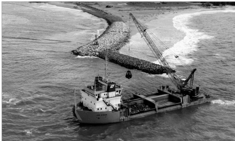
Figure 9.23 Crane mounted on the rock supply vessel Jan Steen (courtesy Van Oord)
