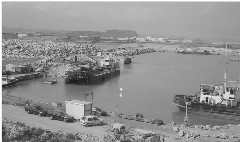
Figure 9.33 General view of Barcelona stockpile where trucks deliver stones to stocks or to a barge for onshore dumping (courtesy CETE de Lyon)
