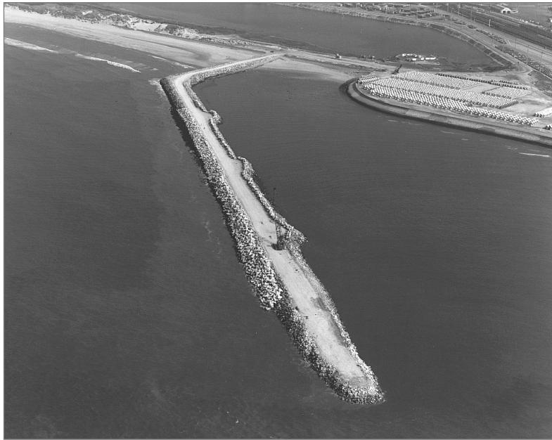
Figure 9.55 Placement of armour layer, showing expansions for turning and passing along the crest of the core (courtesy Van Oord)
