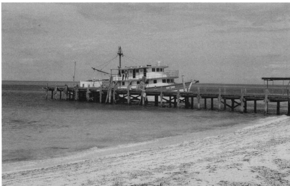
Figure 5.3. A small island jetty. Providing sufficient air gap may not be possible when the level of the quay must be low enough to accommodate smaller vessels (courtesy Doug Ramsay)
