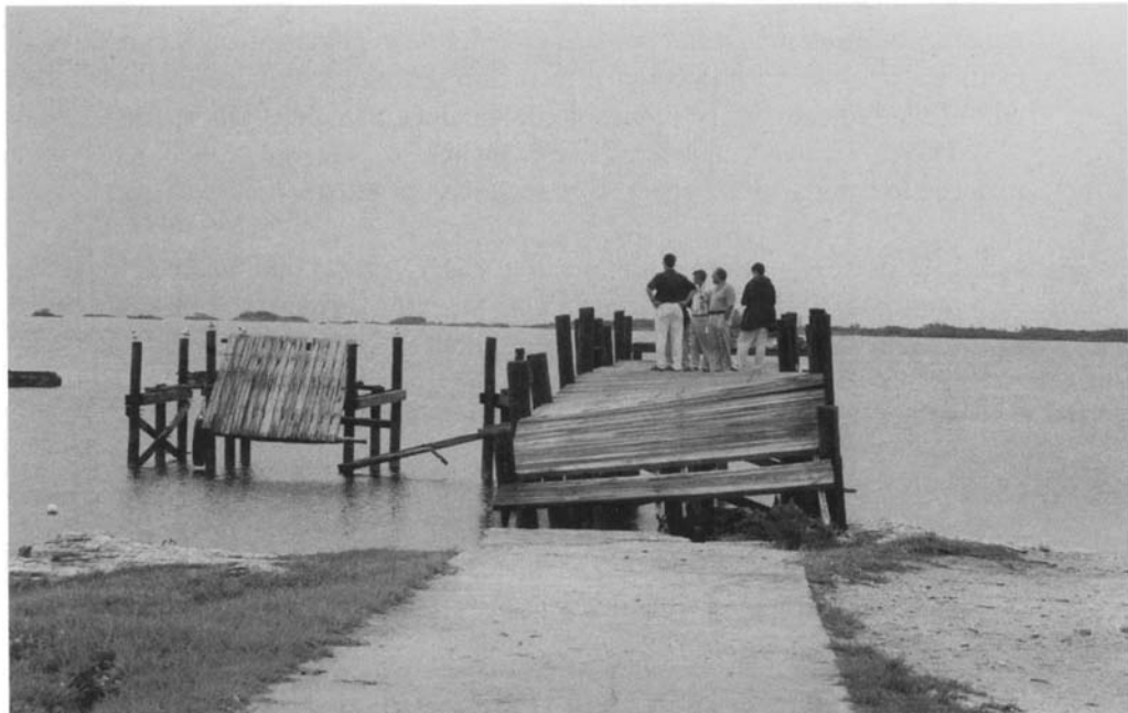
Figure 5.2. Timber jetty damaged due to wave slam underneath deck (courtesy Doug Ramsay)
