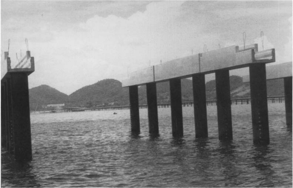
Figure 8.3. Sri Racha Jetty, Thailand, under construction. Use of precast pilecaps allowed infill concrete to be poured without the need for complicated shutters (courtesy Kier)
