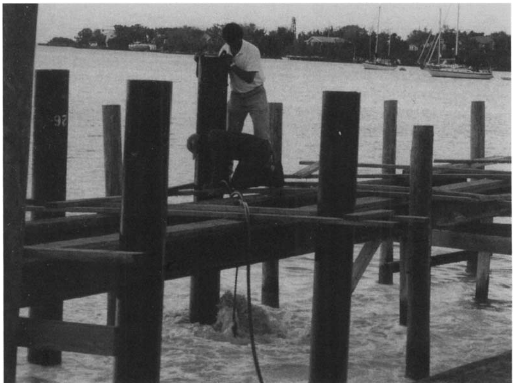
Figure 7.9. Jetty under construction. Pile installation can also cause immediate scour or weaken the soil properties around the pile, resulting in longer term scour (courtesy Doug Ramsay)
