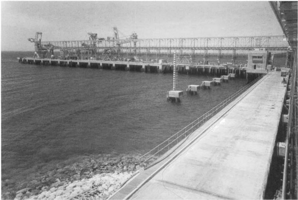
Figure 5.6. Aqaba jetty – bulk loading equipment being erected (courtesy Mott MacDonald and C J Associates)
