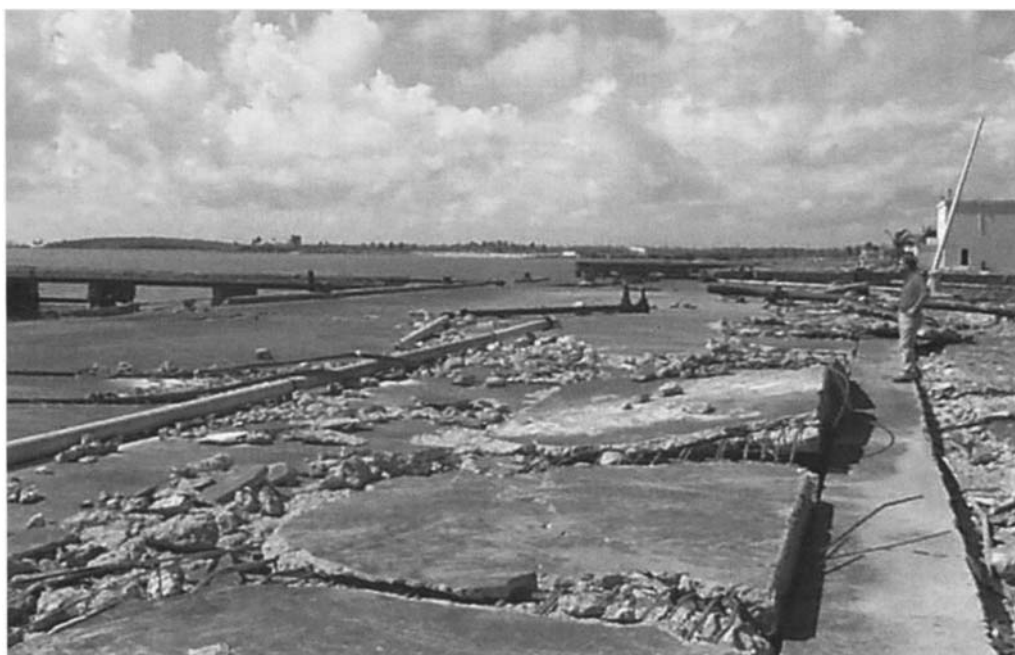
Figure 2.10. Failure of an exposed jetty deck caused by wave uplift forces (courtesy Han-Padron Associates)
