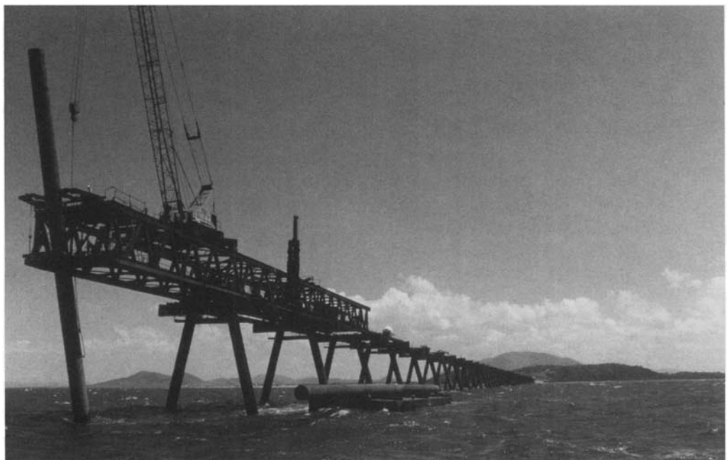
Figure 8.2. A 2.4 km jetty and travelling gantry being constructed at Abbot Point Port Development, Queensland, Australia, to handle 8 million tonnes of coal for export to Japan (courtesy Costain)
