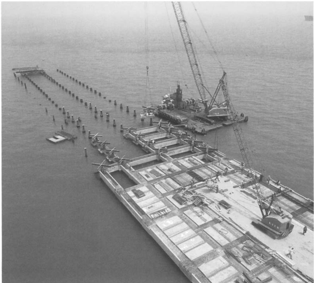
Figure 8.4. Construction of jetty at Banjul, Gambia. The design made use of precast elements to allow modular construction (courtesy Kier)
