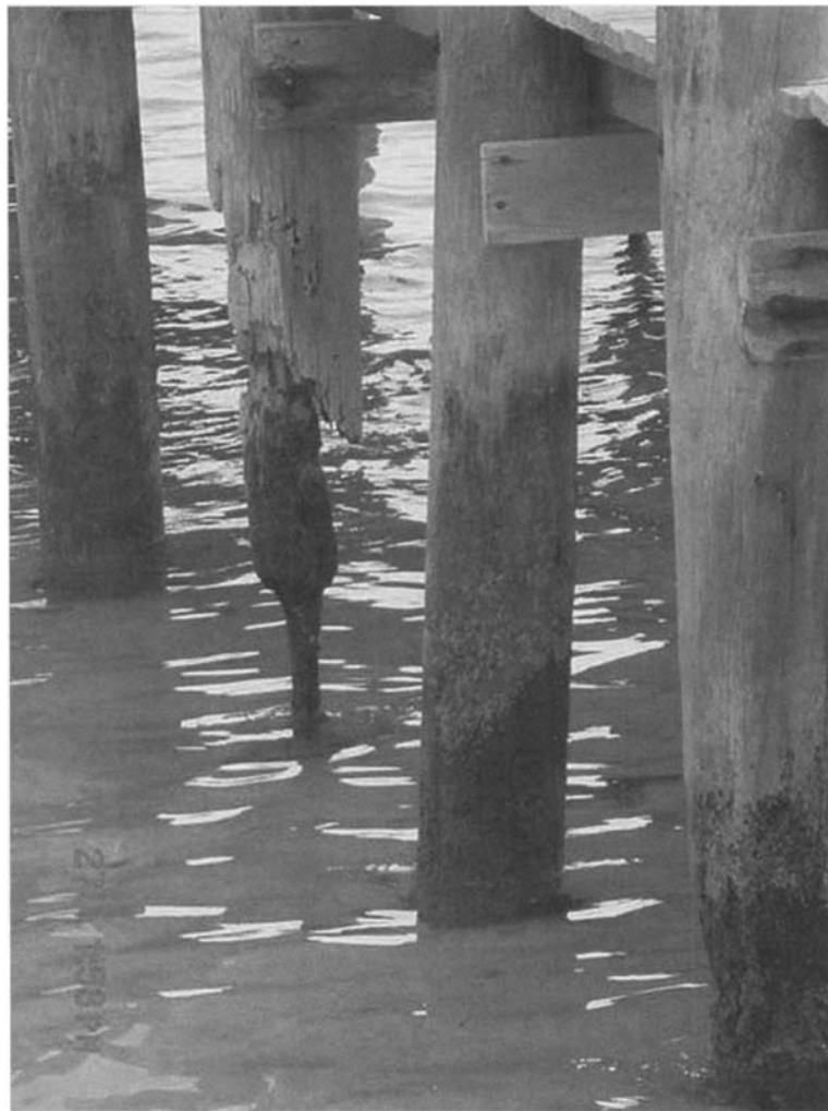
Figure 6.4. Small timber jetty where berthing has damaged a support pile (courtesy Doug Ramsay)
