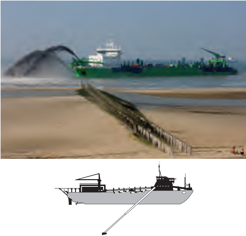
Figure 4.4 A trailing suction hopper dredger pumping sand to the shore for a beach nourishment project.
