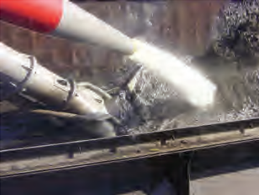
Figure A.40 Jetting water into barge to fluidize dredged material for unloading.
