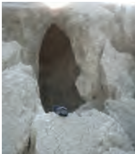
Figure 9.41 Collapsed soil as a result of the intrusion of fresh water (C. de Rooij, Azerbaijan).
