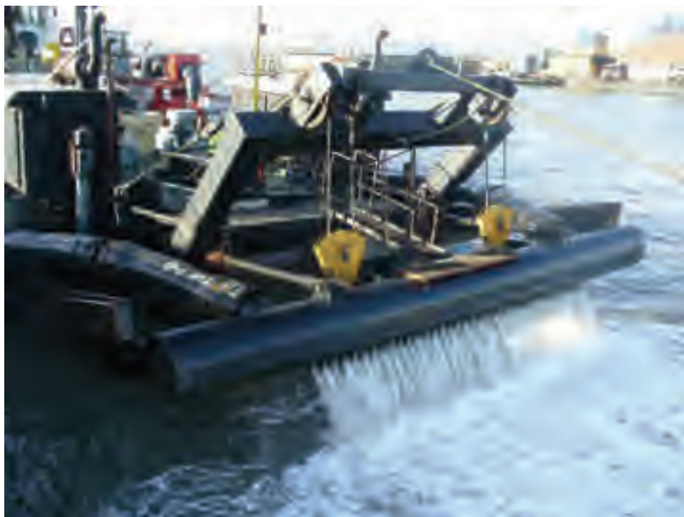
Figure A.28 T-bar (with nozzles) at the end of the ladder of a water injection dredger.
