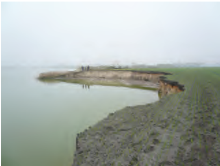
Figure 5.3 Flow slide in inland borrow pit.
