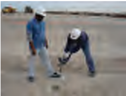
Figure B.28 Making hole for nuclear measurement next to hole of sand cone test.
