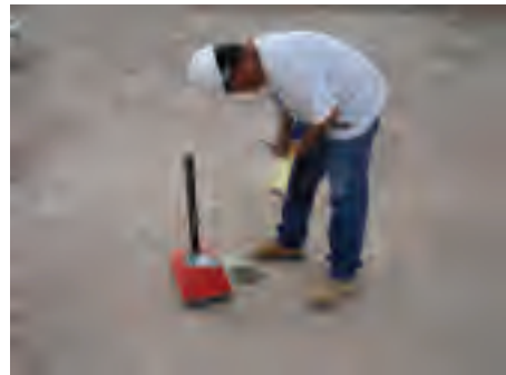
Figure B.29 Nuclear density measurement next to hole from sand cone test.
