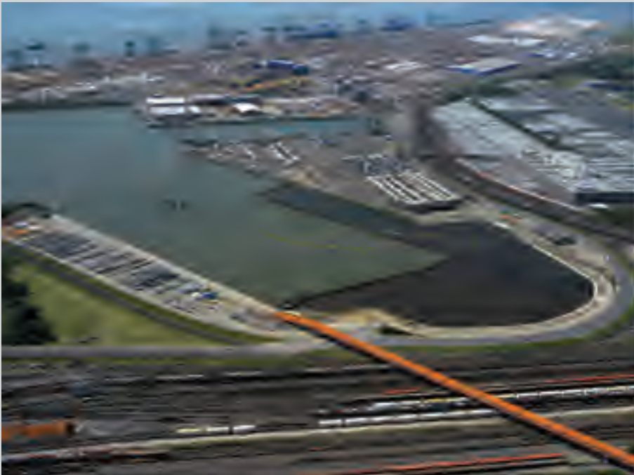
Figure 9.6 Overview Osthafen project during dredging operations: Dredging pontoon in the middle of the basin, floating pipeline and diffuser pontoon discharging the mud in the reclamation area (dark gray area) behind the sheet piled wall.
