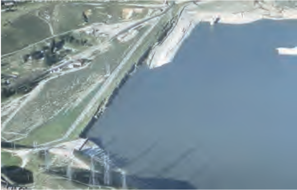
Figure 8.47 The effect of an earthquake on a hydraulic fill, the 1971 failure of Lower San Fernando Dam. Note the paved dam crest road that is mostly now under the reservoir following a liquefaction slide in the upstream shell. (Photograph from Karl V. Steinbrugge Collection, Earthquake Engineering Research Center, University of California, Berkeley).
