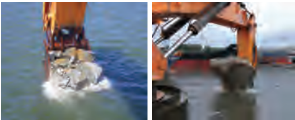
Figure 9.38 Excavation of drilled & blasted rock and removal of boulders in São Francisco do Sul (Brasil).
