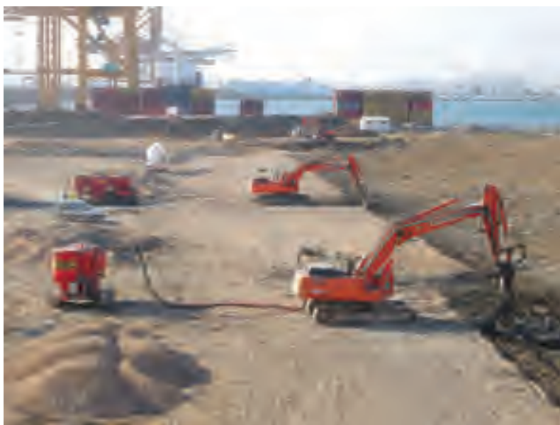
Figure 9.3 In situ treatment of dredged material, Port of Valencia Spain (picture ALLU-Finland).
