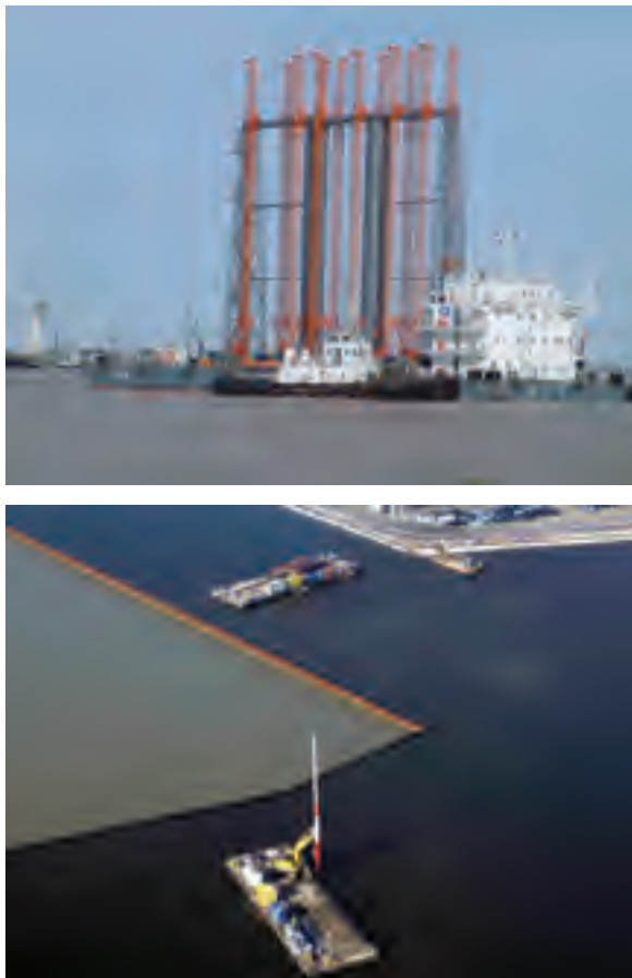
Figure 7.4 Offshore vertical drain installation barge (upper picture, after Yan et al., 2009), and vertical drain installation over water (lower picture) at Osthafen, Bremerhaven, using floating pontoons.
