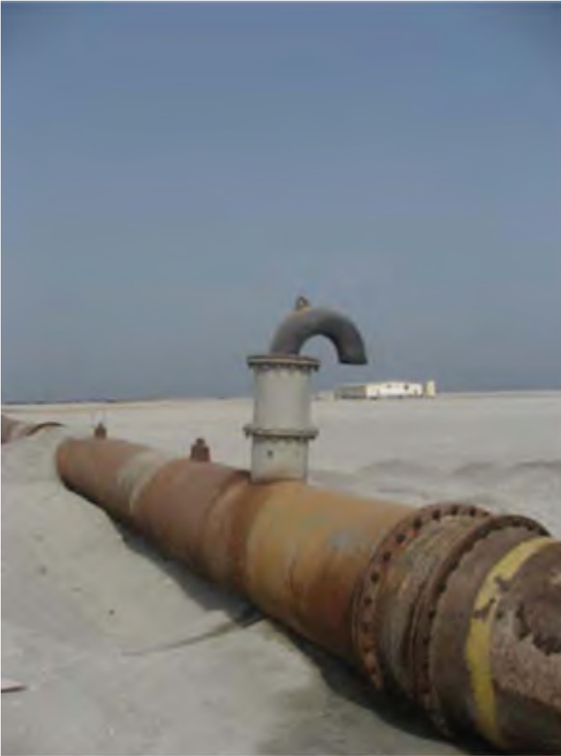
Figure A.34 Snifter on discharge pipe line.
