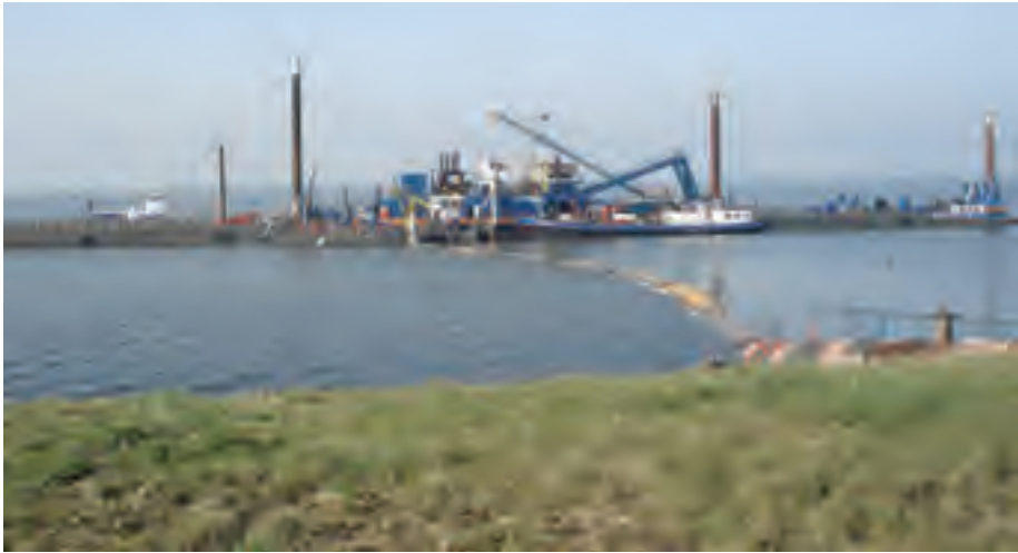
Figure 4.8 A barge unloading dredger which pumps dredged material from a barge alongside the dredger through a discharge pipeline to the shore.
