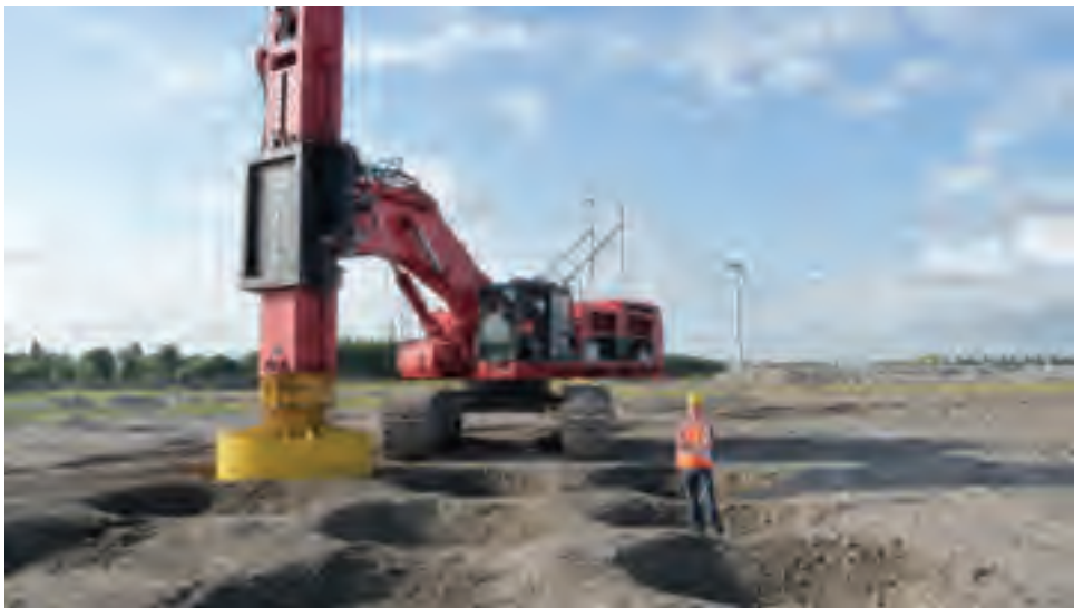
Figure 7.18 A rapid impact compaction machine with 16-ton hammer shifting between impact locations.
