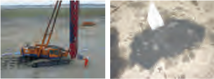
Figure 7.3 Drain installation on land (left) and extracted pore water escaping at top of drain (right).
