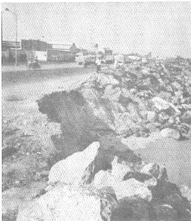
Figure 10-5 Damage of an incorrectly applied revetment
