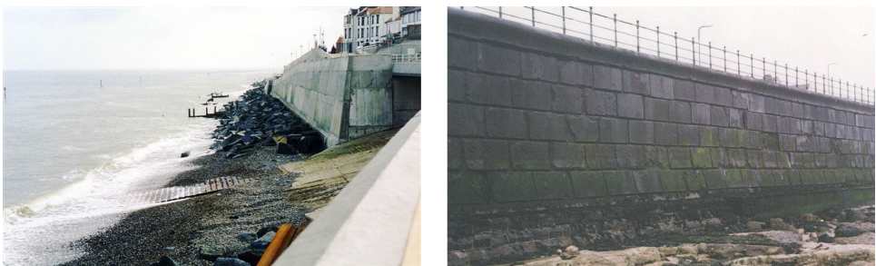
Fig. 16.2. Examples of vertical seawalls: (left) modern concrete wall and (right) older stone blockwork wall.
