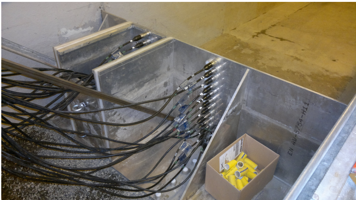
Figure 2.8. Picture of pressure-gauges.
