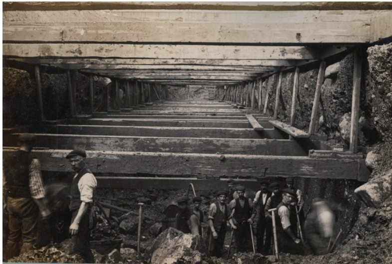
Figure 7.9: Construction pit for a gravity wall in a dry pit, Glasgow 1850 [The Glasgow Story]
