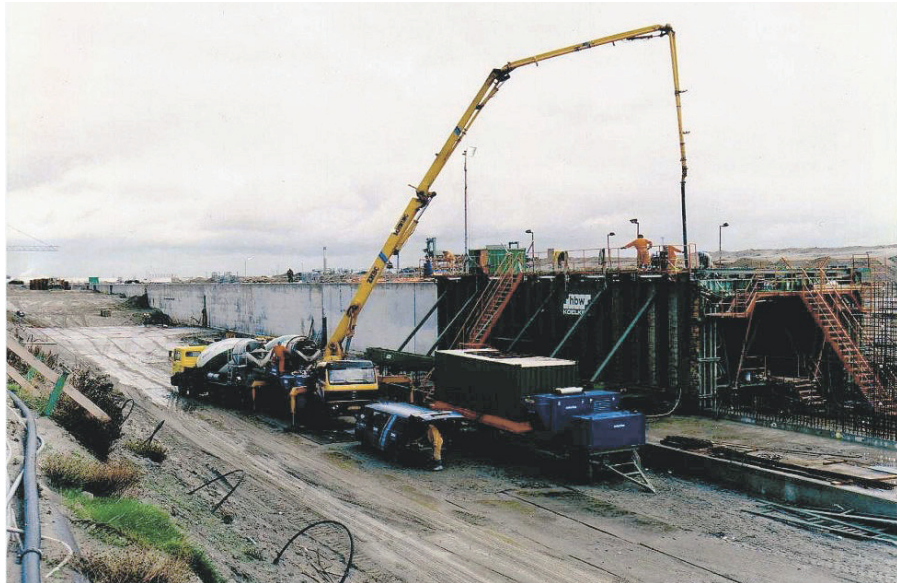
Figure 7.21: The cooling system used in the construction of a concrete quay wall [de Gijt et al 2003]
