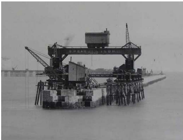
Figure 14. Construction of the south breakwater using a Goliath crane on staging (courtesy of DHB)
