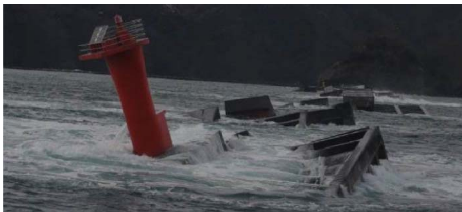
Photo 2. State of damage of North Breakwater
