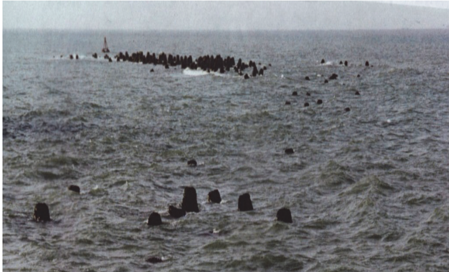
Figure 3.11: Remains (tetrapods) of a breakwater failed by wave overtopping, destroying the rear side of the structure and then a full collapse of the crest. Porbandar, India
