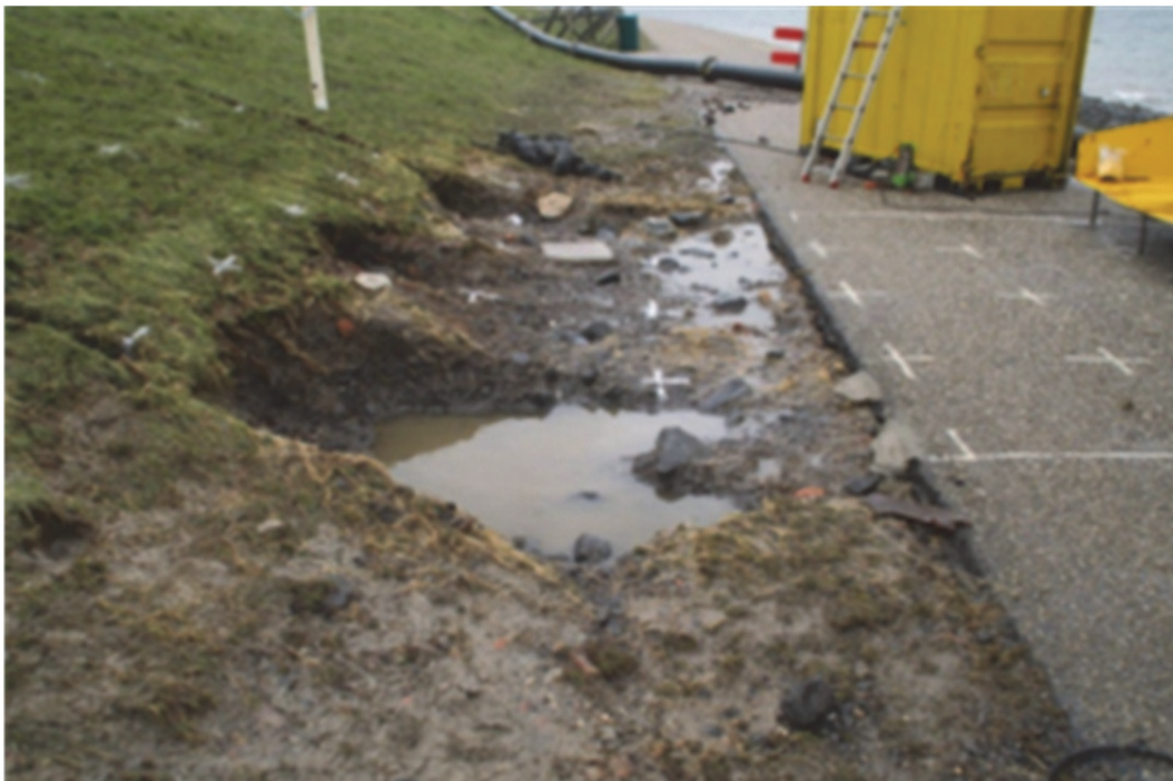
Figure 4.39 Final damage after the pilot run-up test
