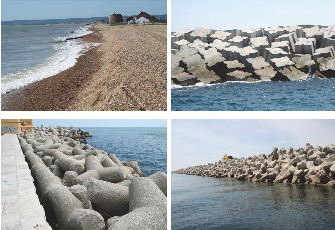
Figure 6.2: Shingle beach and rubble mound structures: shingle beach; antifer cubes; tetrapode; accropode II
