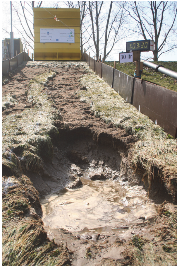
Figure 4.35 Failure of a grass covered sand dike
